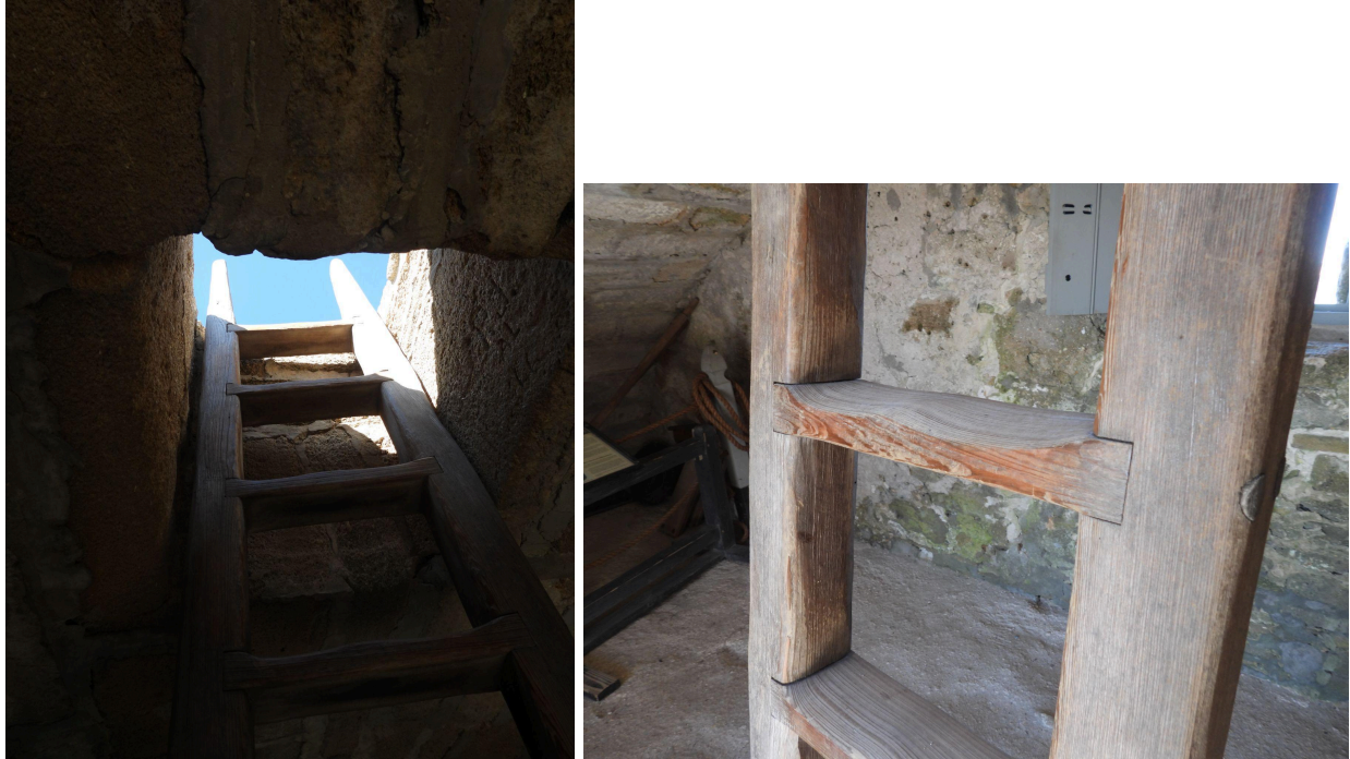
[Figure 44 Sponsor provided photos showing internal ladder placement(left) and ladder details (right)]
